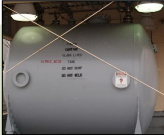
Nitric Acid Tank and Meter
