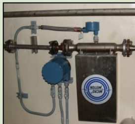
Sulfuric Acid Line & Mass Meter
