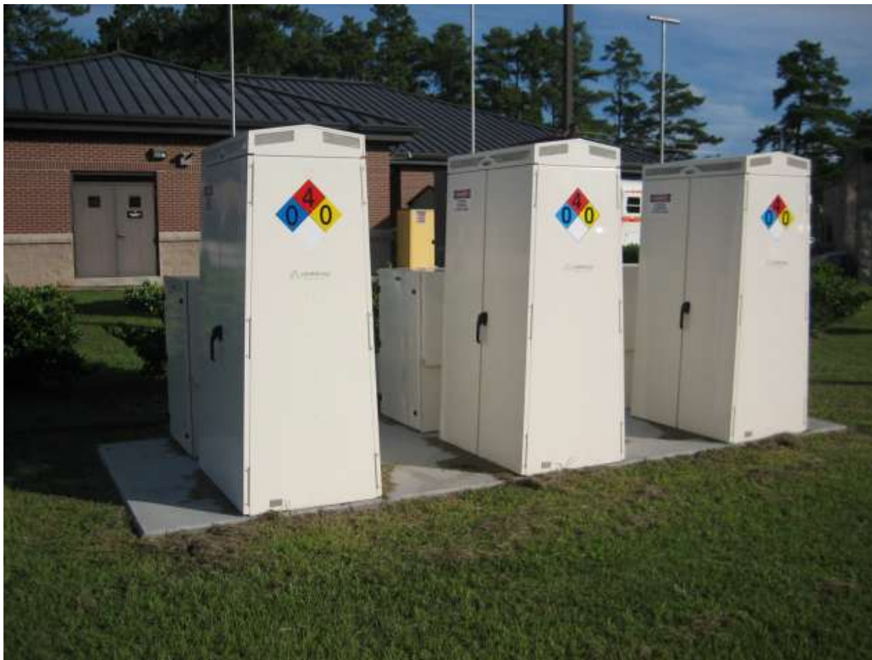
Fuel Cell System Backup for Ft. Jackson Emergency Services Center, April 2009
