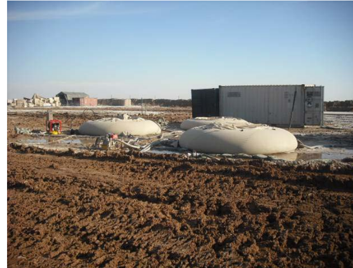
Potable Water Available (Concern is Distribution)
