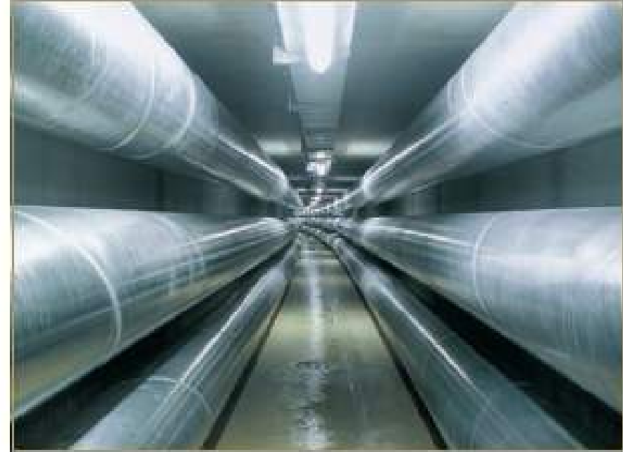
A gas insulated transmission line tunnel in Switzerland.
