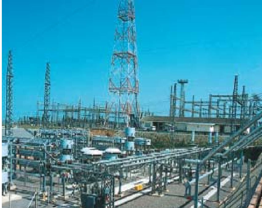
An example of a static VAR compensation installation.
