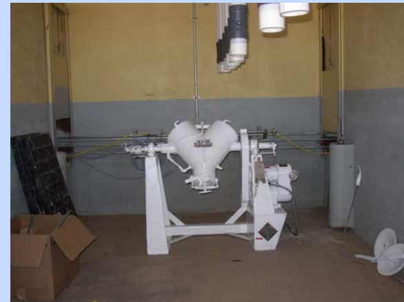
Vacuum cone dryer in bay 6B
